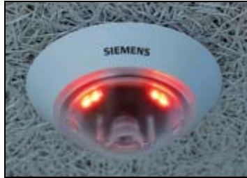
Figure 6-5 Ceiling Mounted Ultrasonic Detector
