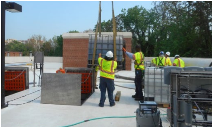
Alexandria Renew team pours sludge with anammox microbes into the centrate pretreatment facility.
