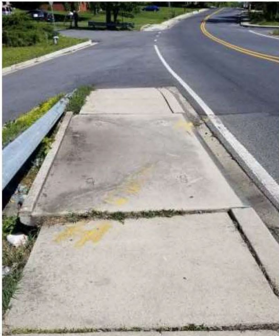
Wide intersection without defined pedestrian path; tripping hazard
