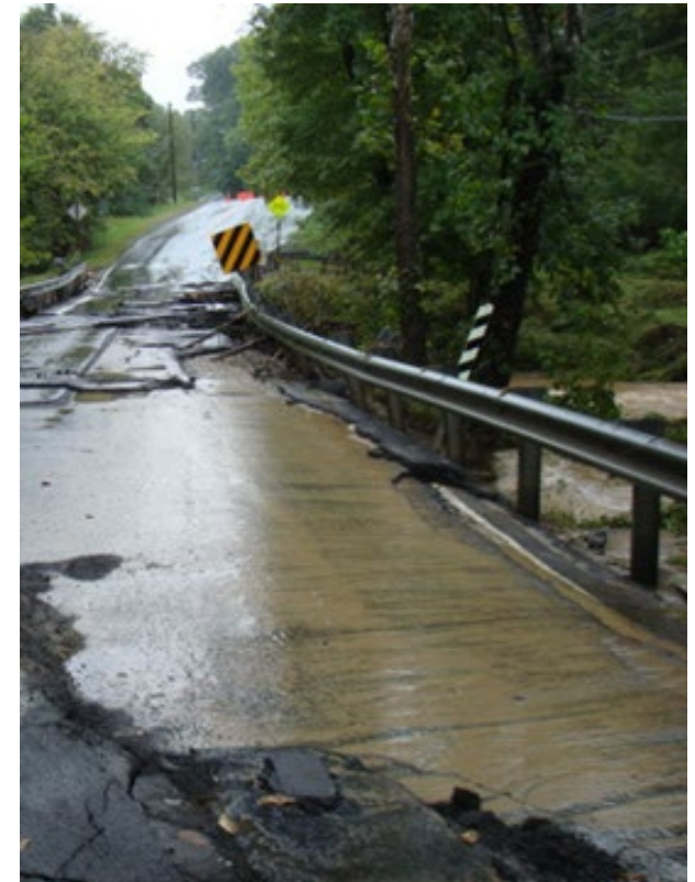
Damage to Hunter Mill Road in Fairfax County from Tropical Storm Lee (Flicker/VDOT, 2011)
