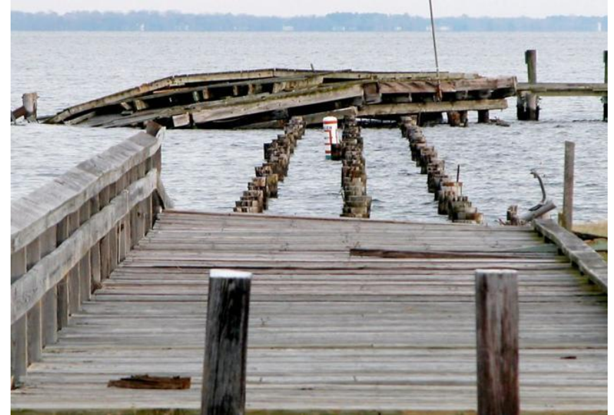
Romancoke Pier in Maryland was destroyed by Hurricane Isabel, 2003. Source: MyEasternShore.
