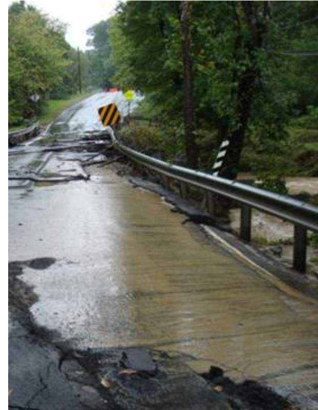
Damage to Hunter Mill Road in Fairfax County from Tropical Storm Lee (Flicker/VDOT, 2011)
