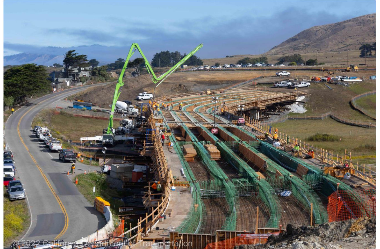
DURING: This photo was taken while construction was underway on the Gleason Beach realignment over Scotty Creek on the Sonoma County coast, which was threatened by rapidly eroding coastal bluffs. (Photo by John Husebay/Caltrans)
