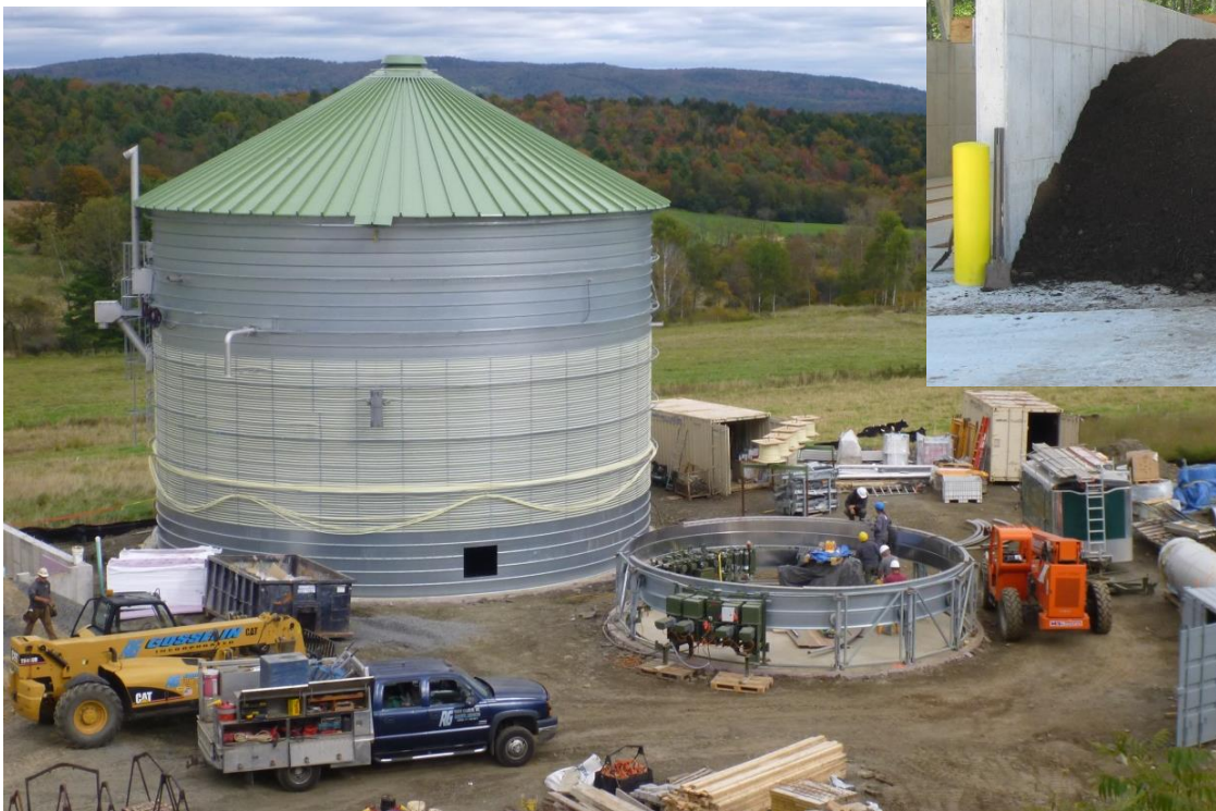
Vermont Technical College's Anaerobic Digester
