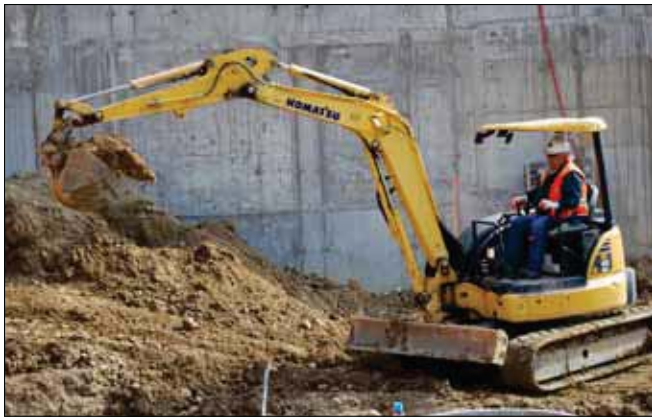
Construction crews are working to improve sewage treatment plants across the Chesapeake Bay region.
