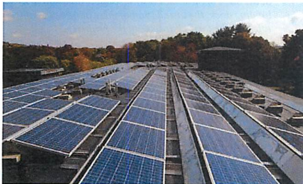
Solar panels installed on the flat roof.
