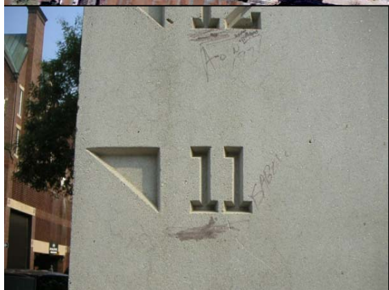
Someone marked the high water point in Old Town Alexandria, VA
