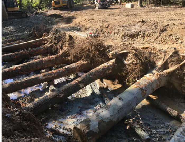
Example of the use of felled trees in stream project in Dewey's Creek Stream Restoration Project in Prince William County. (Prince William County Department of Public Works)
