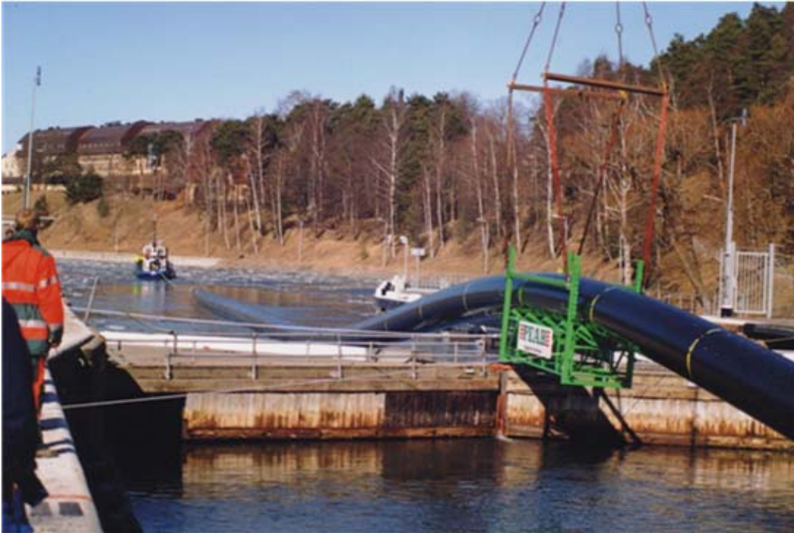
Figure 13. Installation of Polyethylene Pipe for Deep Water Cooling from Lake Mälaren, Sweden
