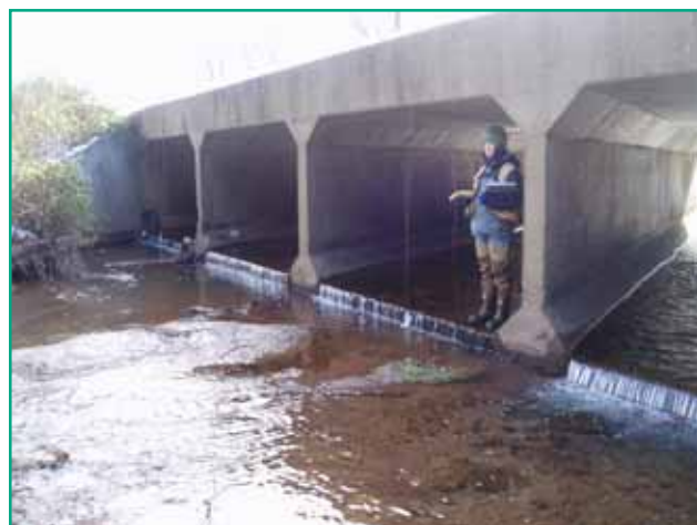
Clarks Run - Saint Clair Lane Quadruple Concrete Box Culvert - Complete Fish Blockage
