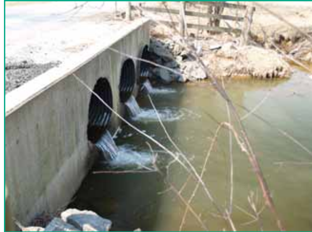
Upper Brens Creek - Complete Fish Blockage - Recent Nixon Road Culvert Replacement Project
