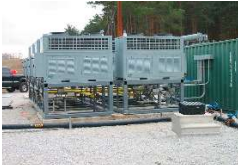
A 200 kW biogas electric unit installation at a landfill in Michigan, 2003.
