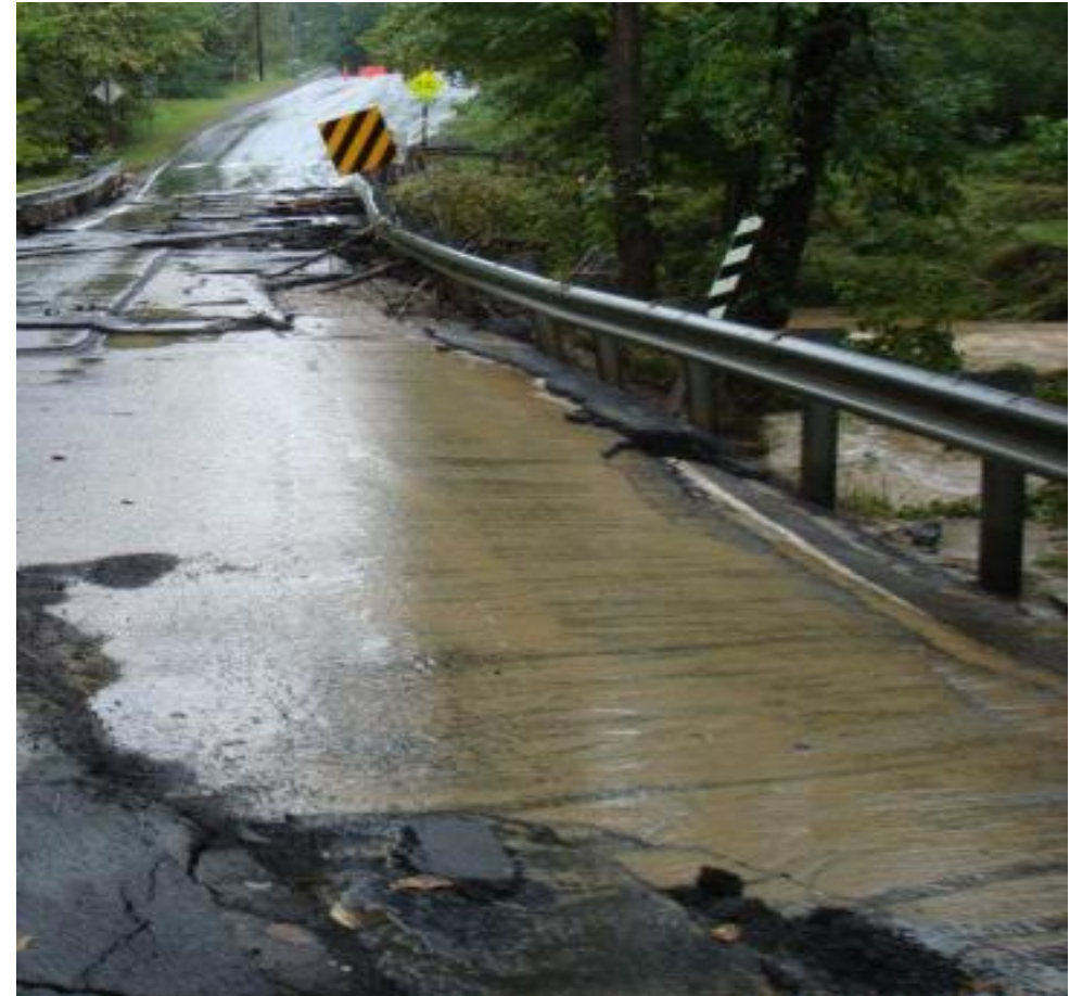
Damage to Hunter Mill Road in Fairfax County from Tropical Storm Lee (2011). Source: Flicker/VDOT
