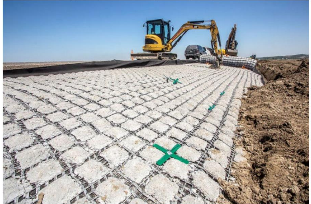
Figure 3 Example of tied concrete block mats in use in western Iowa to protect roadway shoulders from erosion caused by flooding. Source: Iowa Department of Transportation.
