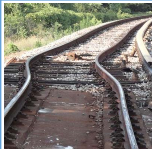
After 10 consecutive extreme heat days this track kink derailed a Metrorail train, July 2012 (no injuries reported) (WMATA).
