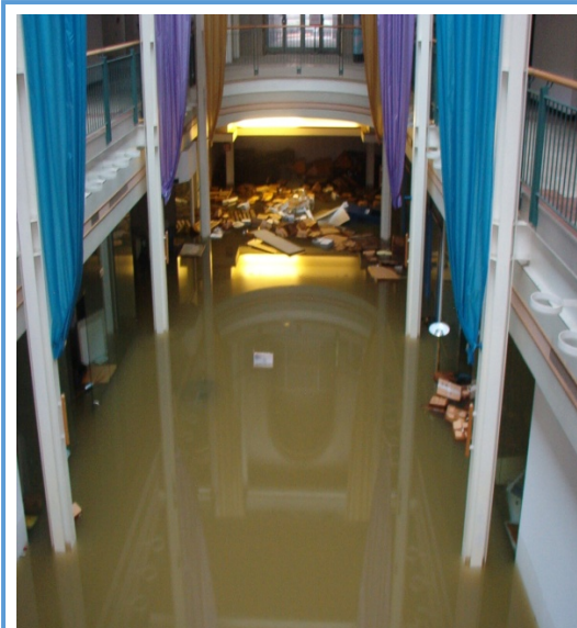
Flood damages the U.S. Department of Justice lobby in June 2006 (DOJ).
