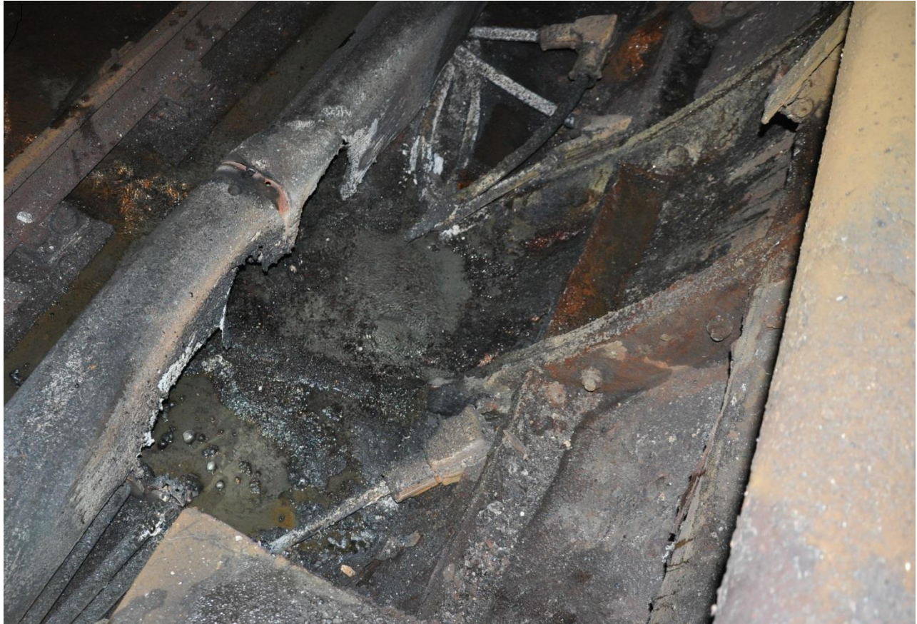
Figure 1. Damage from the arcing incident in the tunnel near L'Enfant Plaza Station.
