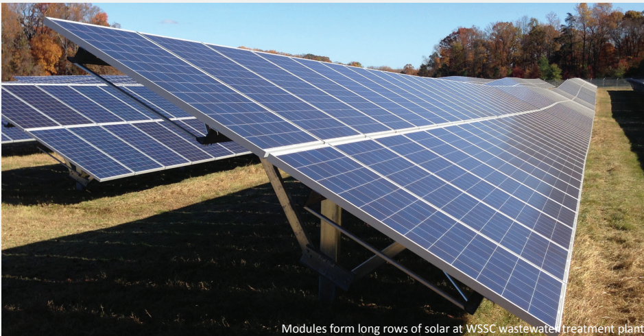
Modules form long rows of solar at WSSC wastewater treatment plant.
