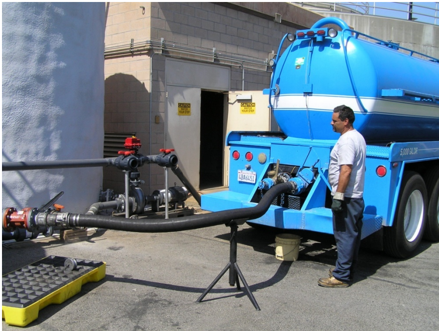
City of Riverside, CA FOG receiving for digester feed
