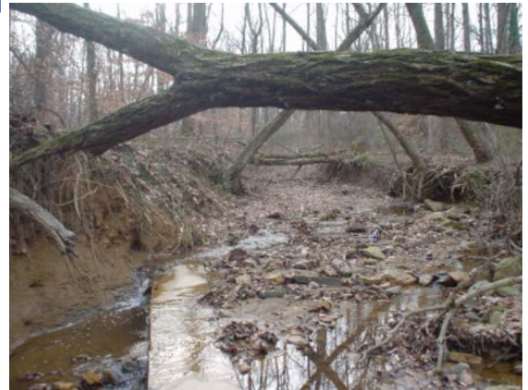
Falling and damaged trees and exposed sewer line in Arlington County
