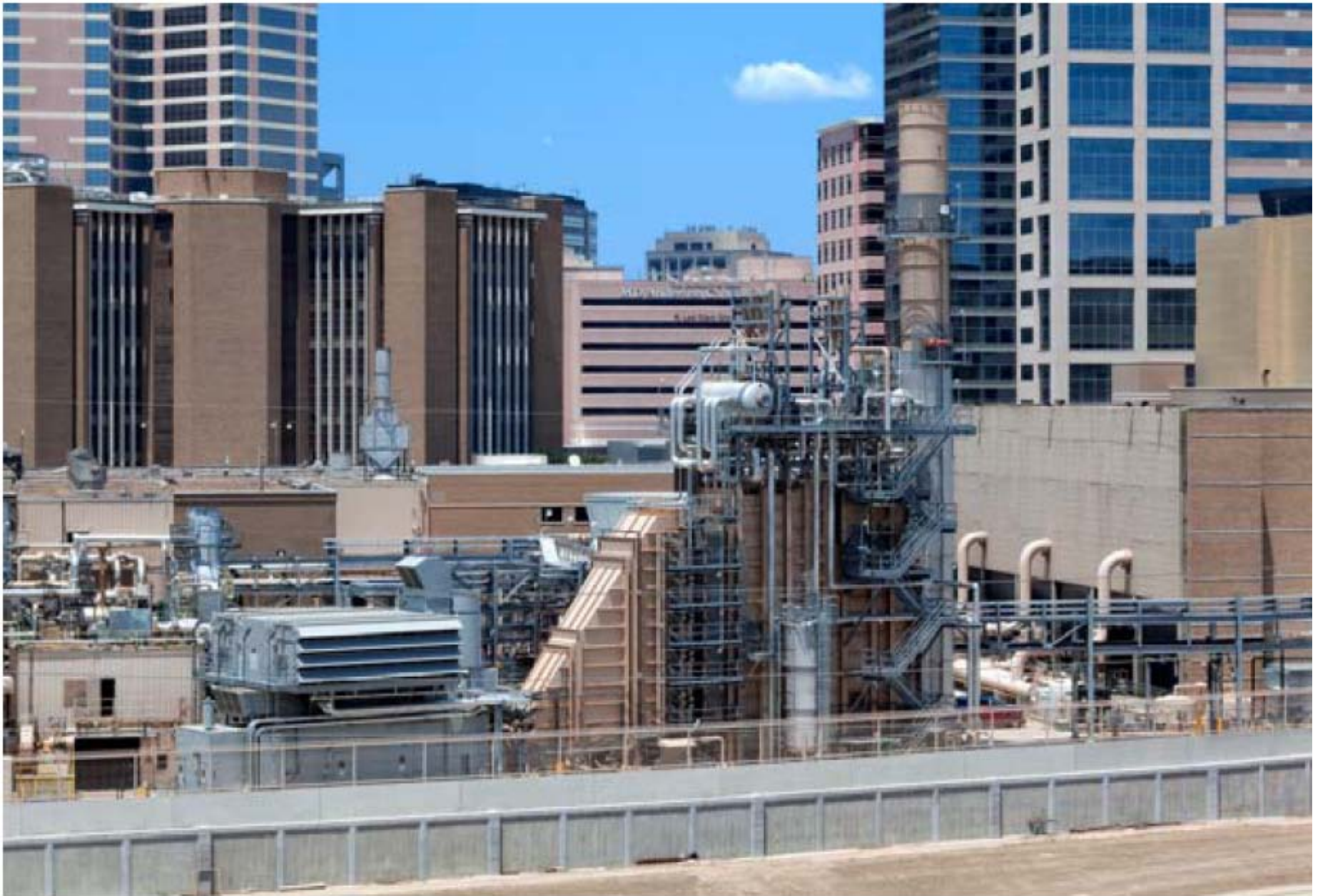
This is the CHP system in the middle of the Texas Medical Center Campus
