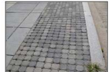
Permeable pavement: District of Columbia
