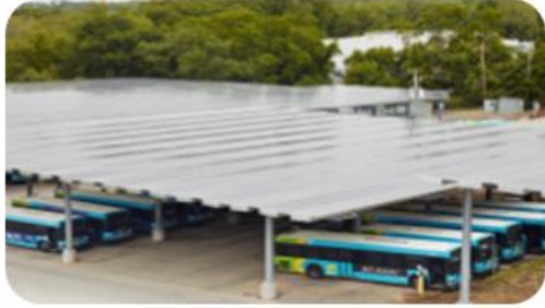
1. 5.5 MW Solar PV Canopy
