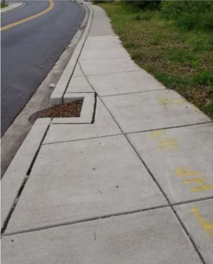
Sidewalk pinch point (manhole)
