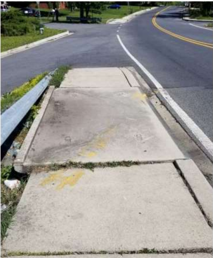
Wide intersection w/o defined ped path Tripping Hazard at storm drain inlet
