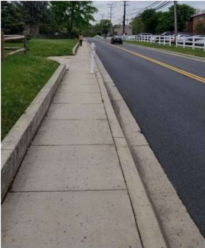
Sidewalk pinch point (mailbox)
