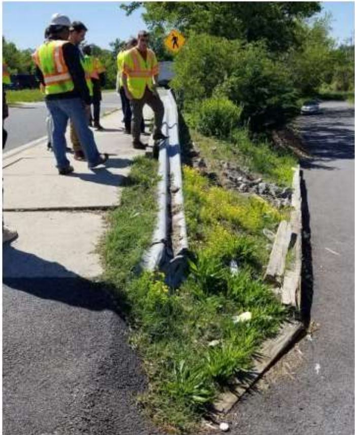
Damaged / collapsed guardrail
