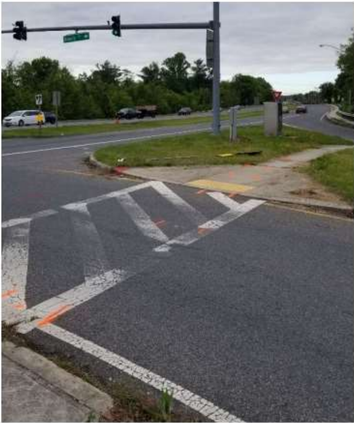
Faded pavement marking
