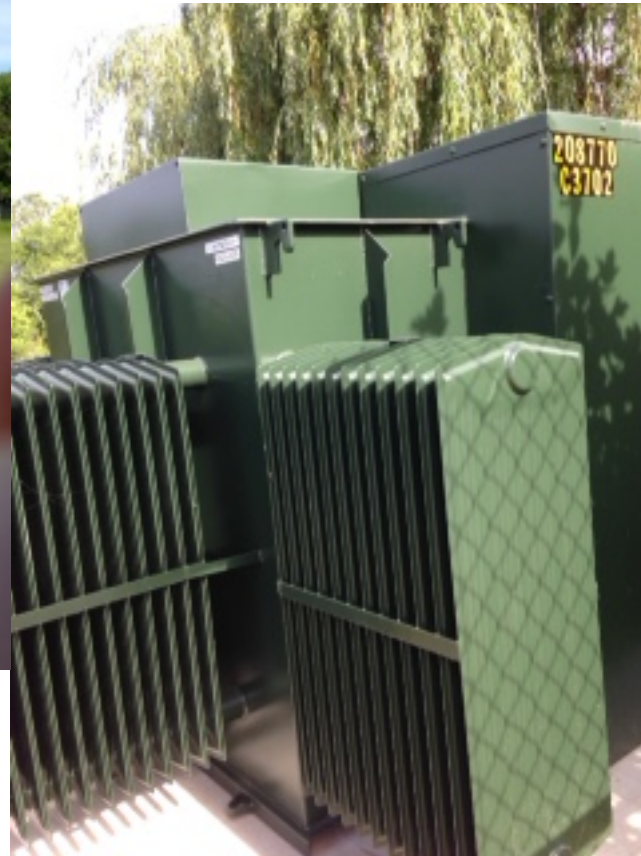
New transformer and electric boxes
