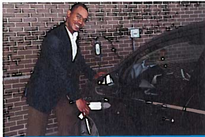
In 2013, the New York Power Authority (NYPA) installed three employee charging stations at its White Plains, New York, facility, as part of its workplace charging pilot program.
