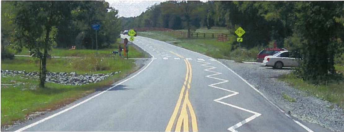
Figure 5: The existing parking and portions of the vegetation are limiting sight lines between trail users and motorists below the clearance areas recommended by AASHTO
