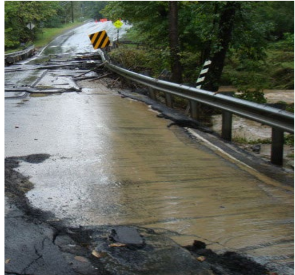
Figure 1. Damage to Hunter Mill Road in Fairfax County from Tropical Storm Lee (2011). Source: Flicker/VDOT
