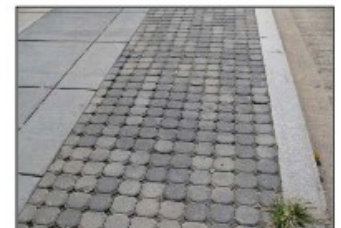
Permeable pavement: District of Columbia
