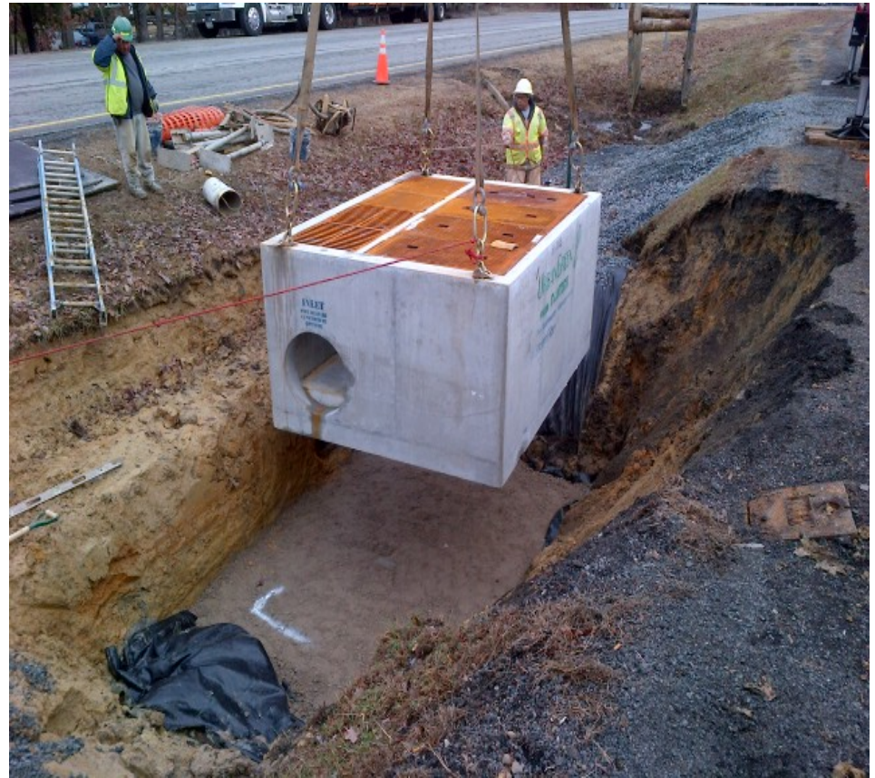
Storm Filter BMP on Old Bridge Rd project
