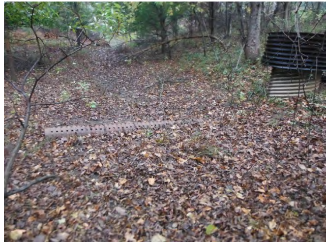
Figure 4 - Hunt Ridge pond bottom facing west at low flow perforated Outlet pipe.
