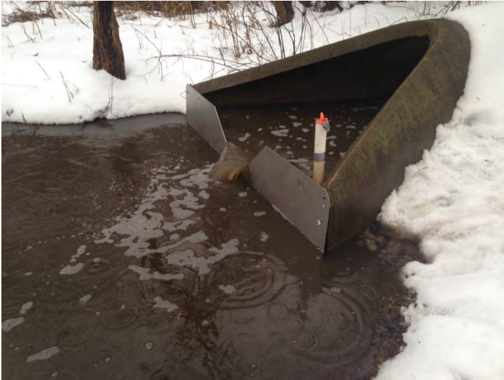
Worthington: Inlet weir
