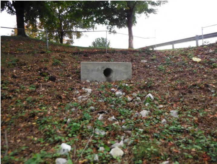
McCormick: Inlet A
