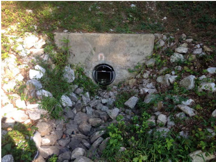
McCormick: Inlet B
