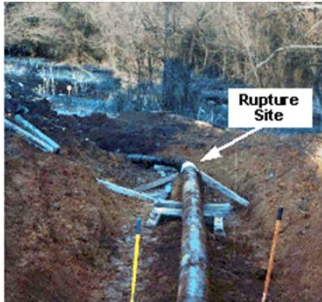
Colonial Pipeline Rupture
