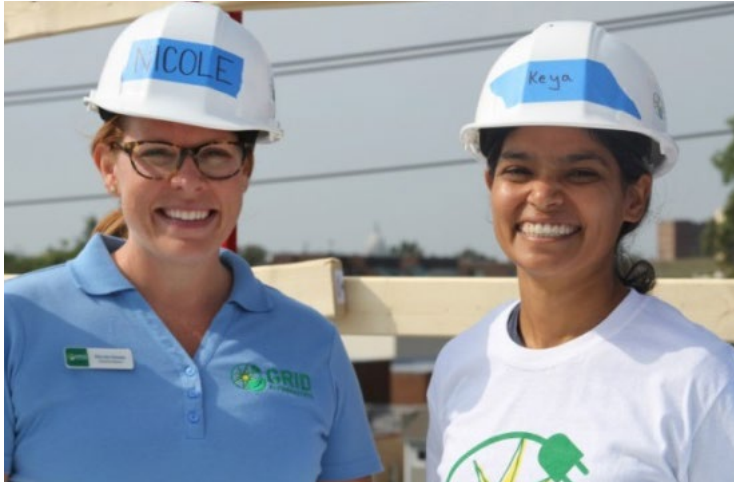
Nicole Steele, GRID Alternatives Mid-Atlantic Executive Director, and Keya Chatterjee, U.S. Climate Action Network Executive Director, on the roof during GRID's Executive Women's solar install on Habitat for Humanity passive homes in Washington, D.C.
