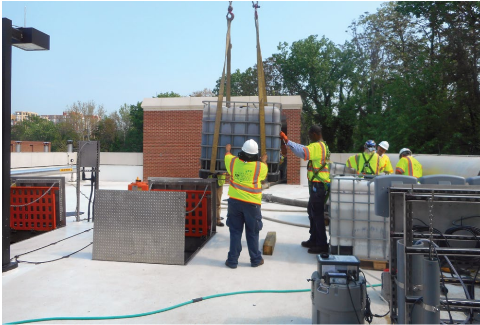
Alexandria Renew team pours sludge with anammox microbes into the centrate pretreatment facility
