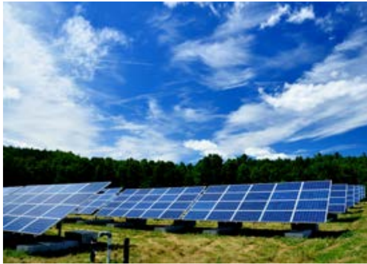
Figure 6-1. A 2.3 MW solar energy system sited on top of a closed municipal landfill in Easthampton, Massachusetts (Source: Flickr / Massachusetts Department of Environmental Protection (CC BY 2.0))
