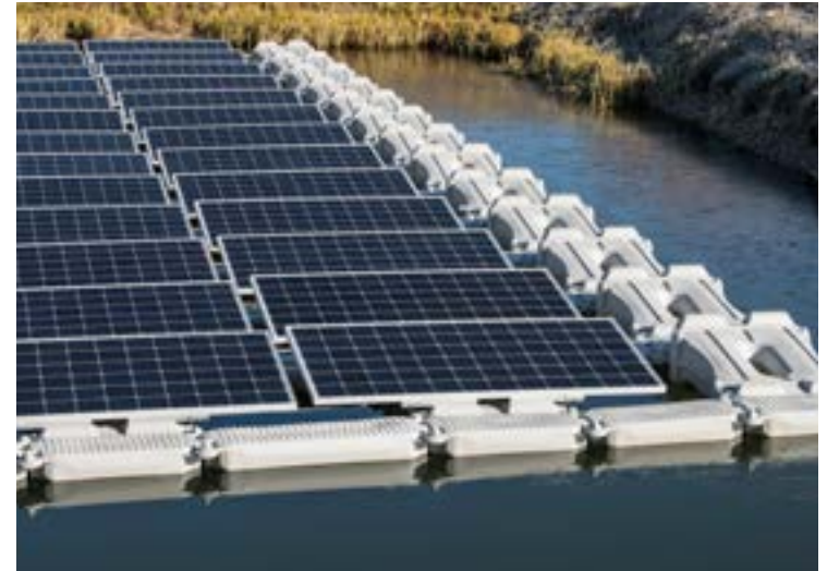
Figure 8-2. A floating PV system on a retention pond at a municipal water treatment facility in Walden, Colorado (Photo by Dennis Schroeder / NREL)
