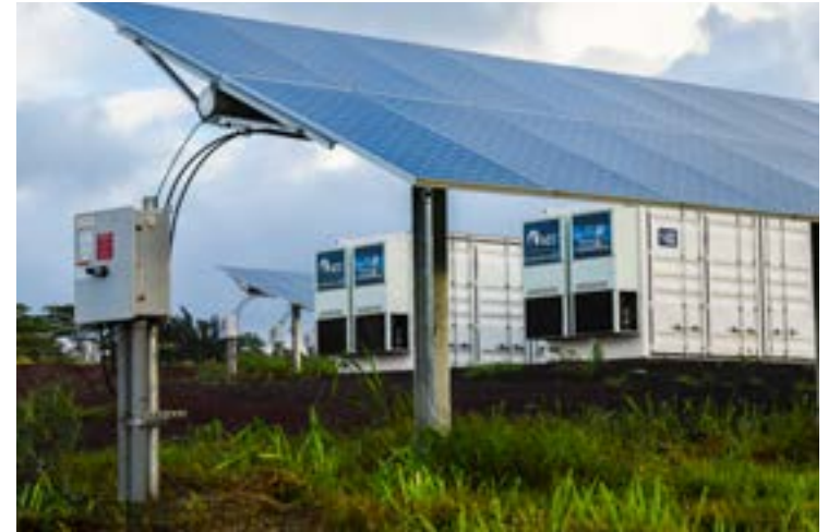
Figure 8-1. The AES Lawai Solar Project in Kauai, Hawaii (Photo by Dennis Schroeder / NREL)
