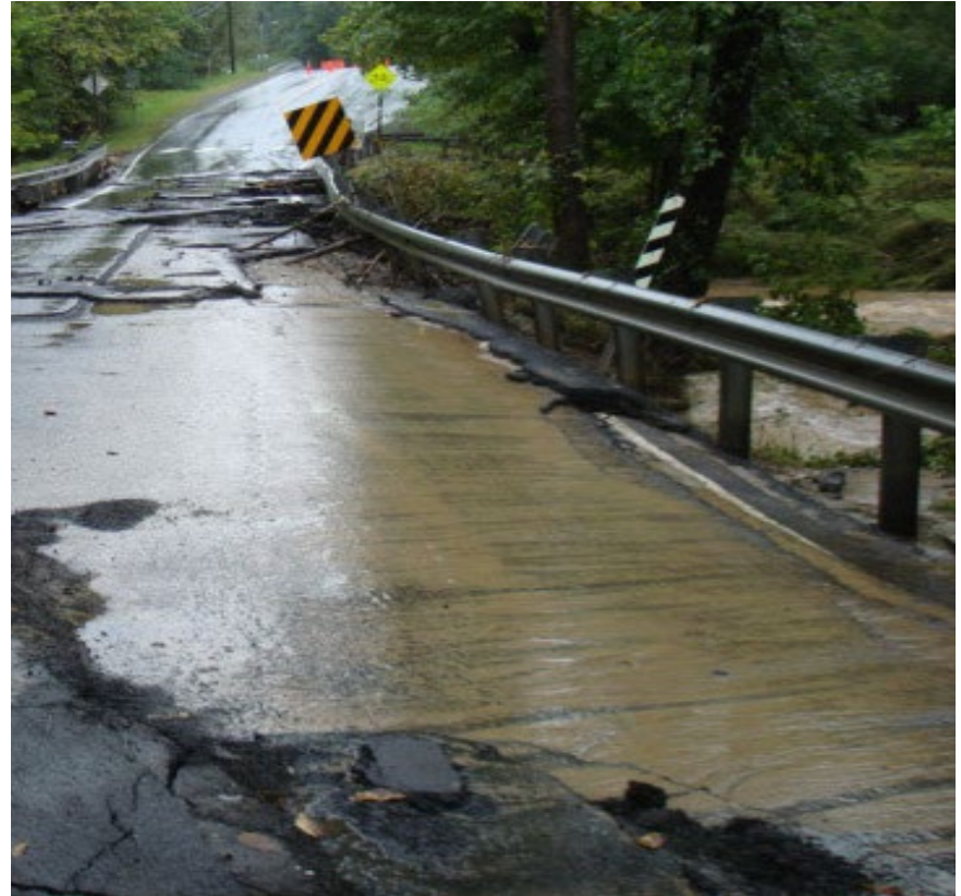
Figure 1. Damage to Hunter Mill Road in Fairfax County from Tropical Storm Lee (2011). Source: Flicker/VDOT
