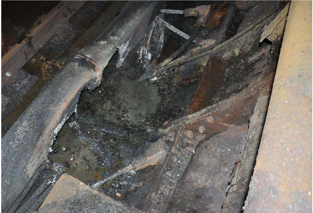
Figure 1. Damage from the arcing incident in the tunnel near L'Enfant Plaza Station.
