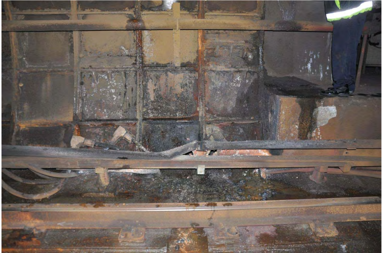
Figure 2. Damage from the arcing incident in the tunnel near L'Enfant Plaza Station.
