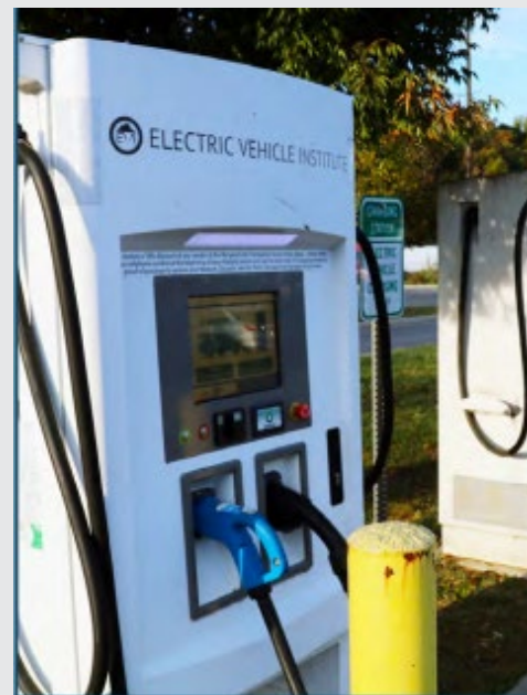
Figure 13: EV charging station (MDOT).
