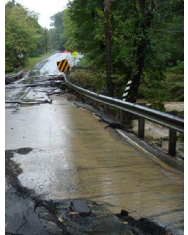
Damage to Hunter Mill Road in Fairfax County from Tropical Storm Lee (Flicker/VDOT, 2011)
