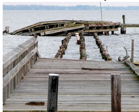
Figure 29. Hurricane Isabel destroyed Romancoke Pier in Maryland.
