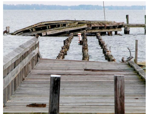
Figure 29. Hurricane Isabel destroyed Romancoke Pier in Maryland.
