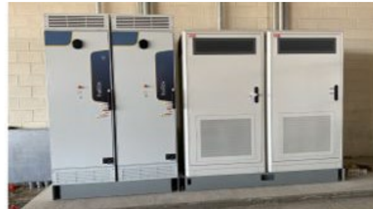
Charger cabinets and pantographs installed at Shepherd Parkway
