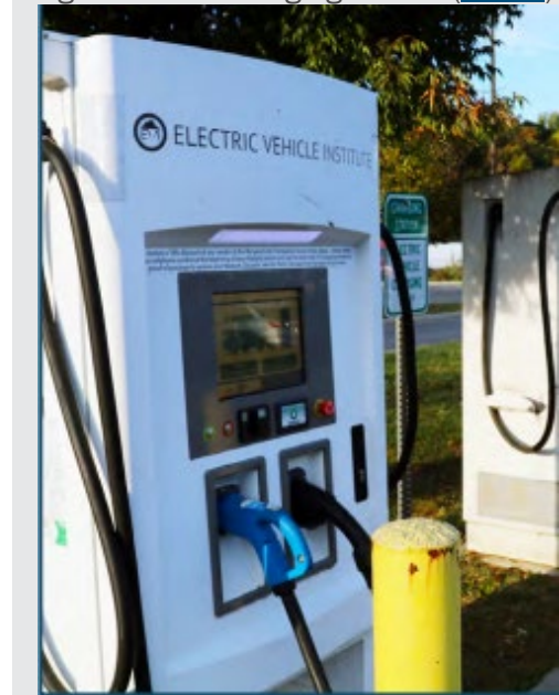
Figure 13: EV charging station ( MDOT ).
