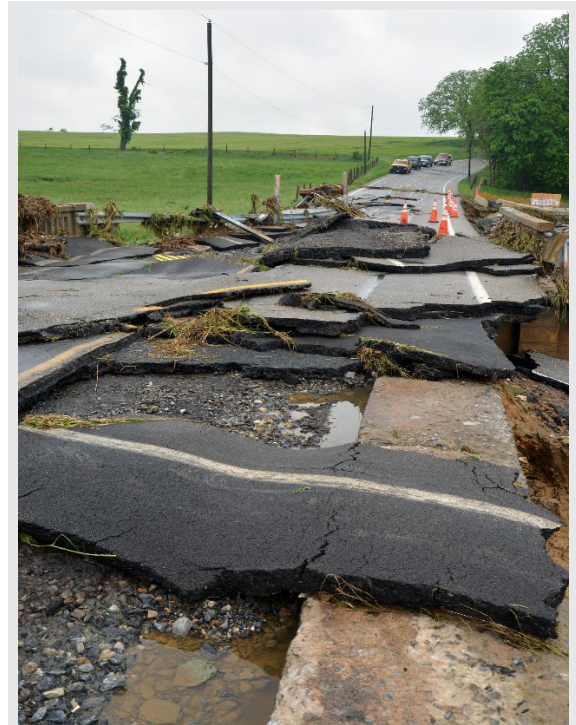
Road damage from flooding event, 2018 (Maryland GovPics/ Flickr ).
