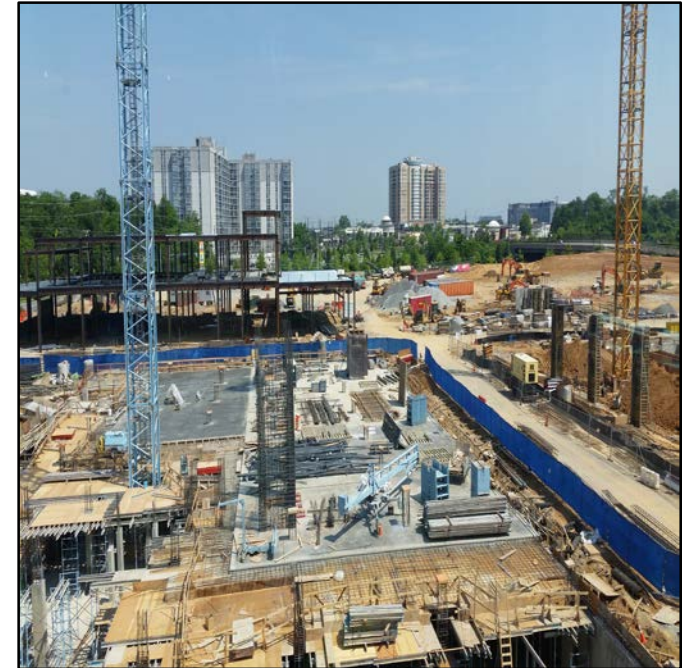
Pike and Rose TOD under construction near White Flint Metrorail, Montgomery County, MD
