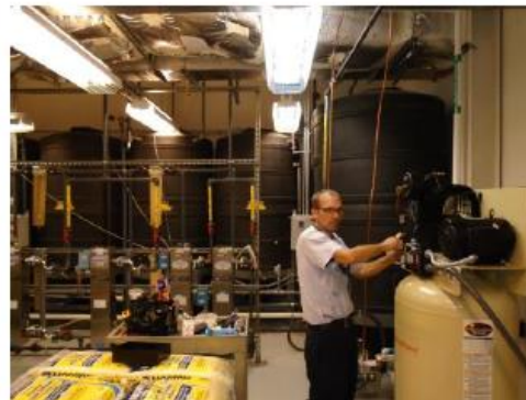
Well Water System
