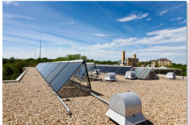
4600 Connecticut Solar Water Heating System
