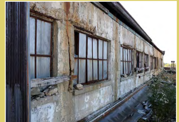
Top: Exterior after conversion Above: Before conversion Credit: TWG Development / Indiana Landmarks
