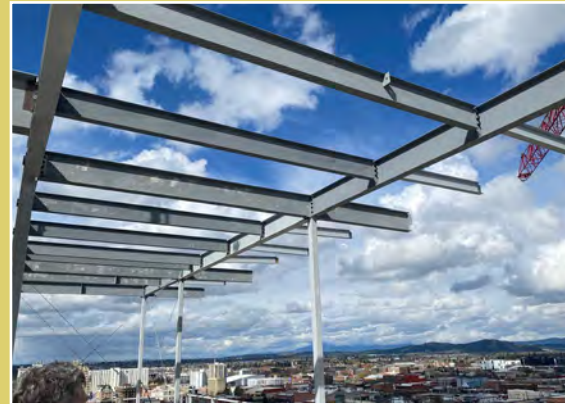
Top: During conversion Above: During conversion, view from rooftop Credit: Brumback Real Estate
