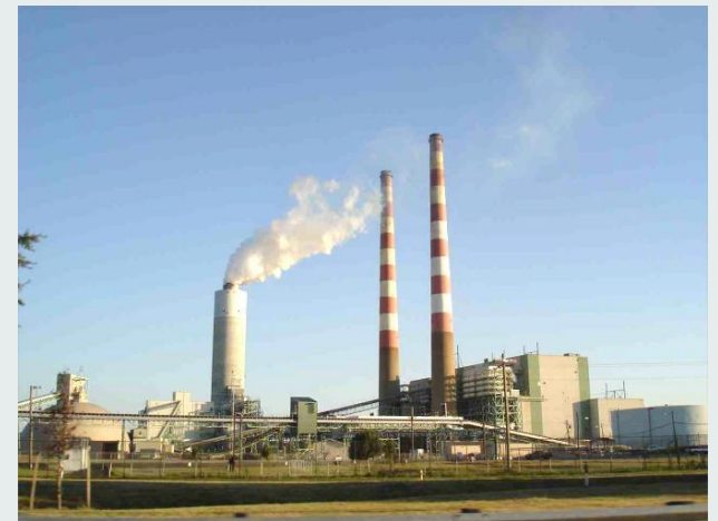
Wet Scrubber Installed at Morgantown Coal Plant - 2009
