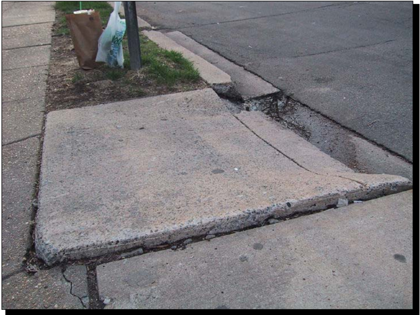
Settling problem at curb ramp
