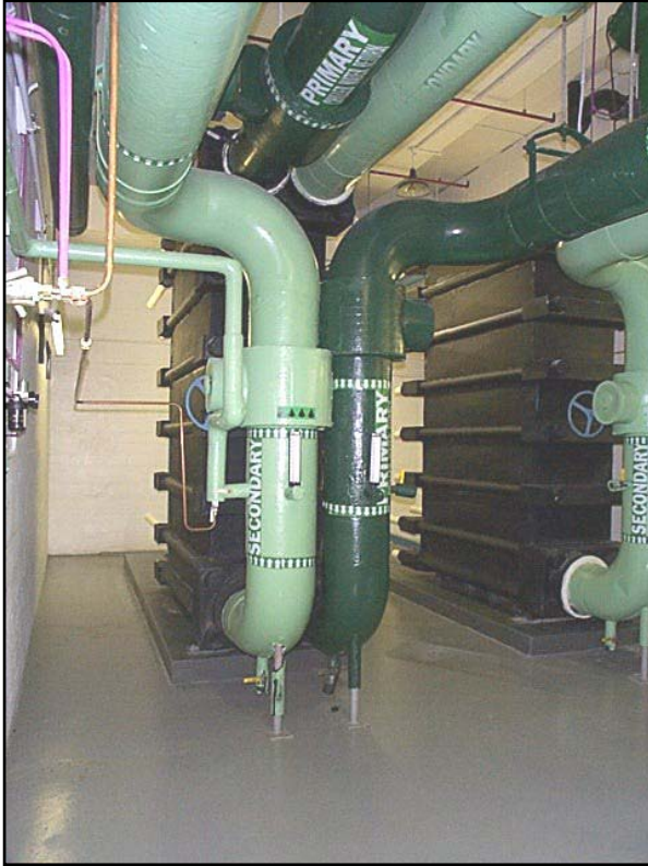
Figure 7. Heat Exchanger Used to Transfer Thermal Energy to Building System
