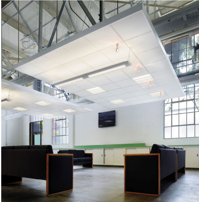
Electrified Ceiling Grid
